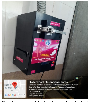
Sanitary napkin Incinerator in ladies toilet MIST MAIN BLOCK GROUND FLOOR
