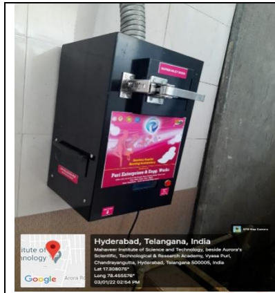
Sanitary napkin Incinerator in ladies toilet MIST BLOCK SECONDFLOOR
