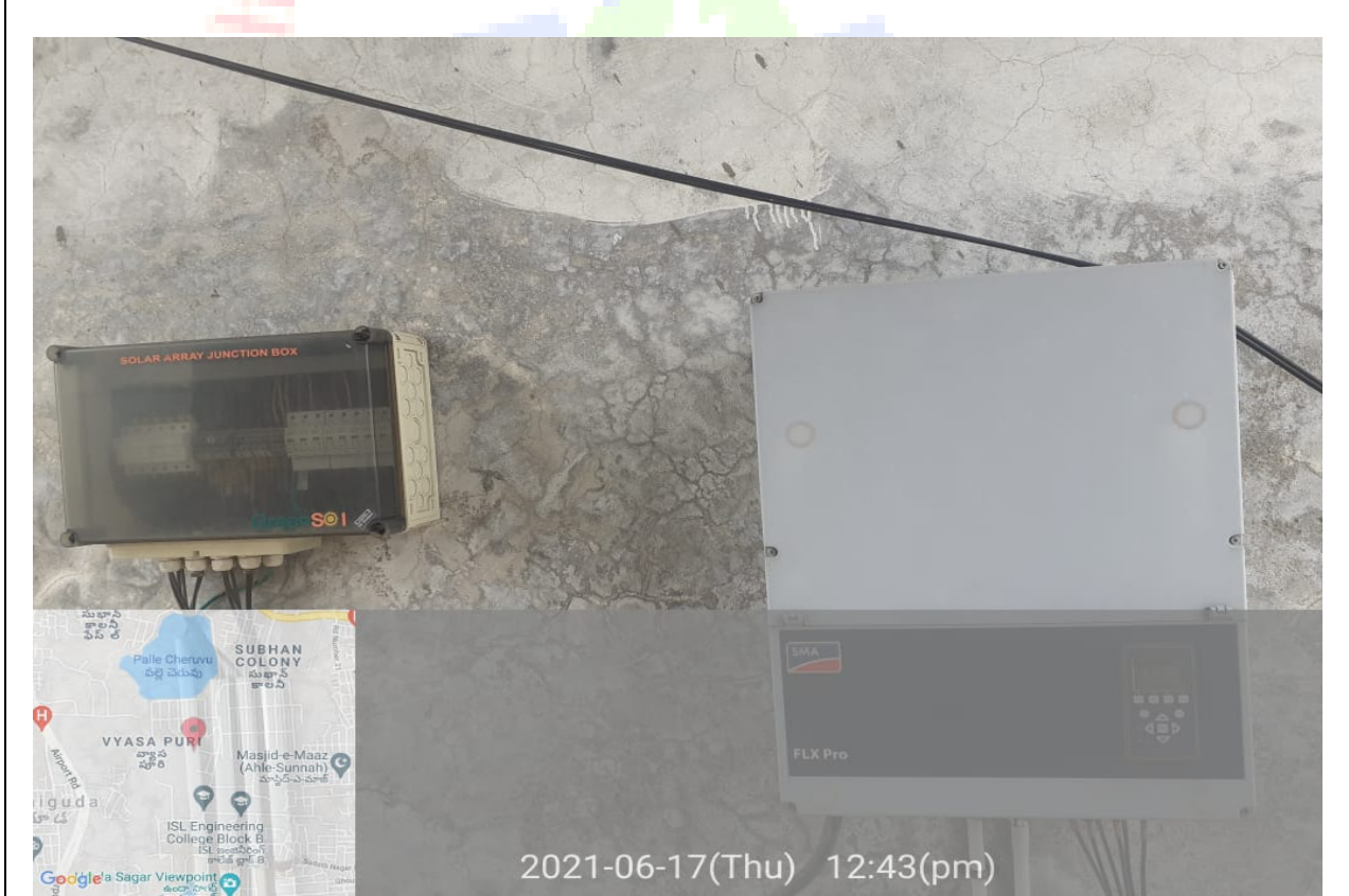
Solar PV Inverters
