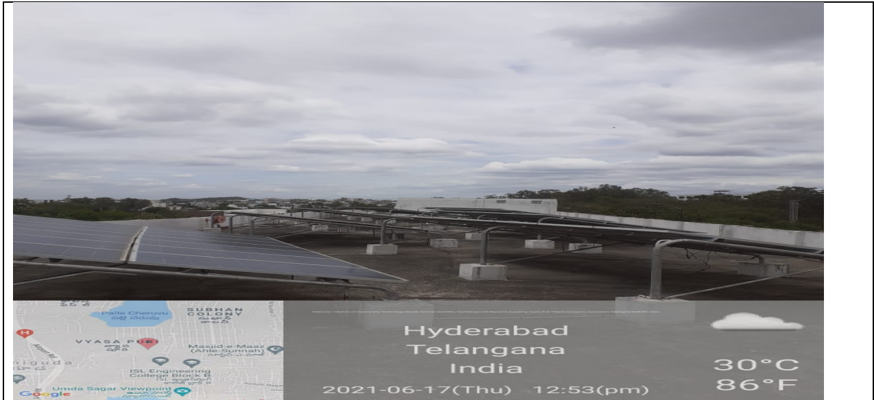
Solar PV Panels on roof top
