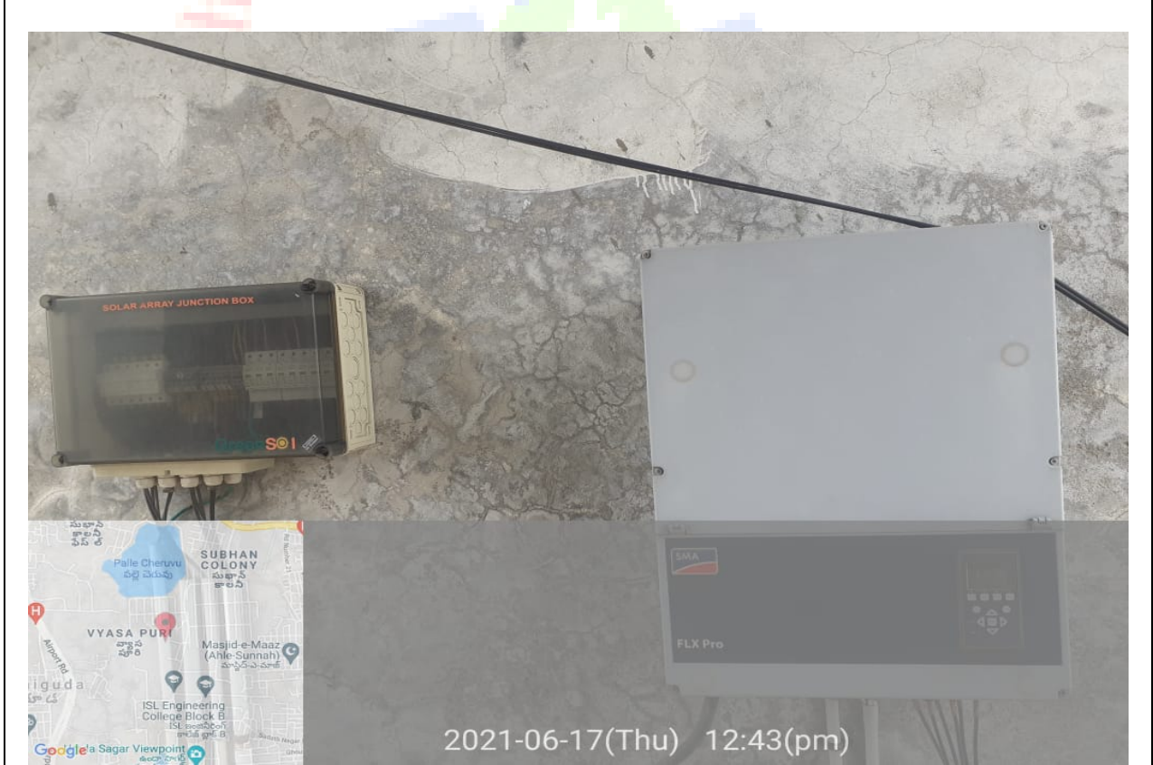
Solar PV Inverters
