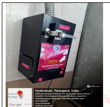
Sanitary napkin Incinerator in ladies toilet MIST BLOCK SECONDFLOOR
